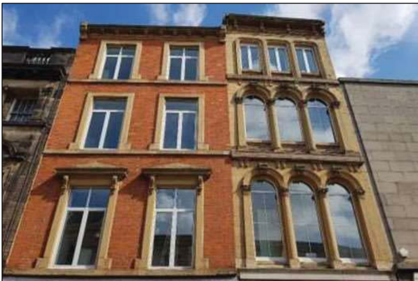
Figure 59: Unsympathetic replacement windows later rectified through planning enforcement action.
