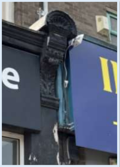
Figure 50 - Retained console brackets to No 121 Spring Bank (Author, 2023)
