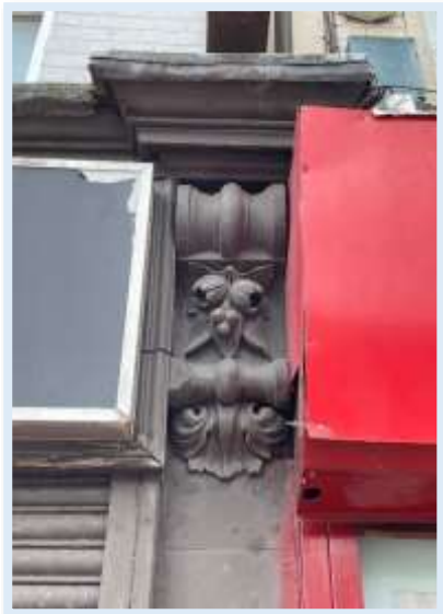
Figure 51 - Retained console brackets to No 151 Spring Bank (Author, 2023)
