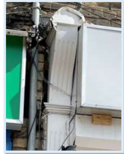
Figure 60 - Retained console brackets to No 102 Spring Bank (Author, 2023)
