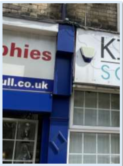
Figure 54 - Possible retained console brackets (behind box-out) to No 122 Spring Bank (Author, 2023)
