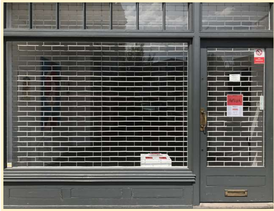
Figure 70 -Example of an internal lattice grill shutter to a restored shopfront (Shopfront, 2023)
