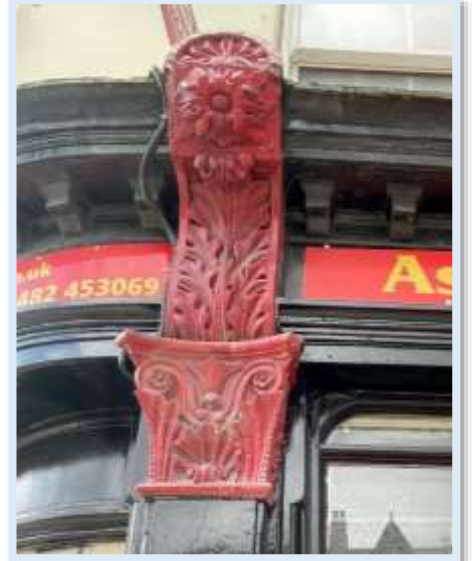
Figure 52 - Retained console brackets to No 169 & 121 Spring Bank (Author, 2023)
