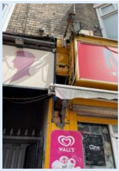
Figure 56 - Retained console brackets to No 114 Spring Bank (Author, 2023)
