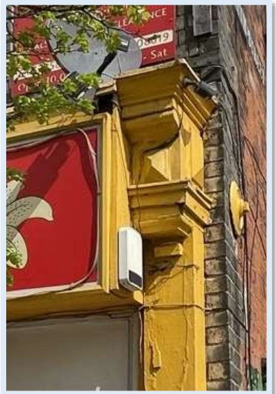
Figure 55 - Retained console brackets to No 121 Spring Bank (Author, 2023)
