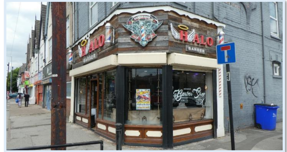
Figure 91 No.414 - Positive element of a timber shop front but with poor quality advertisements.
