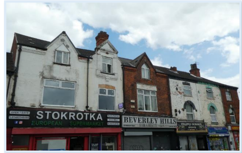
Figure 123 Poor quality windows in the Stepney area.
