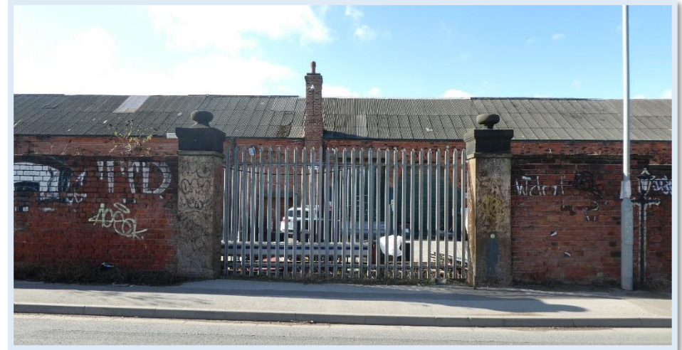
Figure 86 - Use of security fencing is not in keeping with the boundary wall of the Grade II former Sculcoates Goods Shed.
