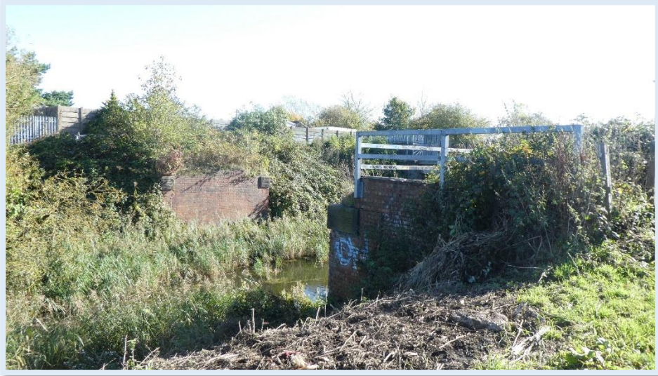
Figure 32 Late 19th century footings of the former railway bridge at Bridlington Avenue.
