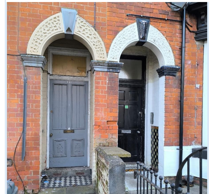
Figure 22. Original door with decorative panels and moulding. Porch featuring encaustic floor tiles and Victorian wall tiles. (Source: Author, 2025)
