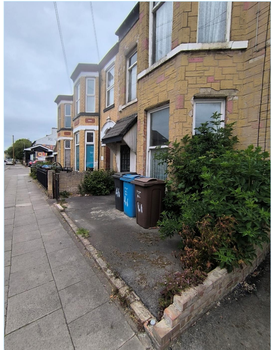
Figure 15. Complete loss of boundary treatment is a negative aspect in the CA.
