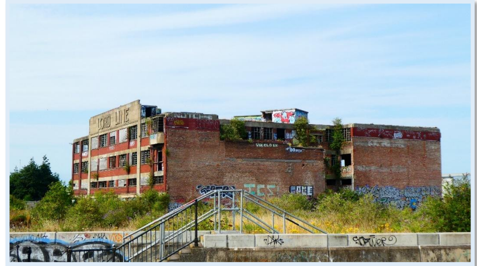
Figure 28 The Lord Line Building in 2024, following the demolition of the J. Marr Building.
