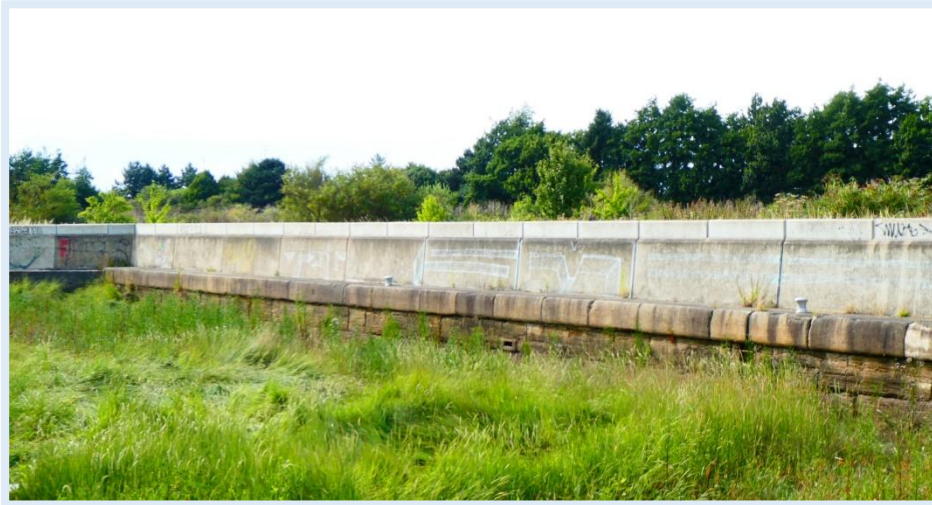
Figure 35 - Enclosure of the lock by the flood wall.
