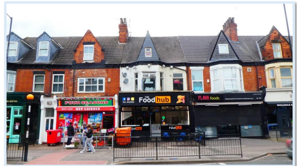
109 - Poor quality advertisements and roller shutters at Nos.65-69, and alterations to dormers.
