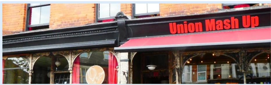
122 - Unauthorized canopies at Nos.22-24.
