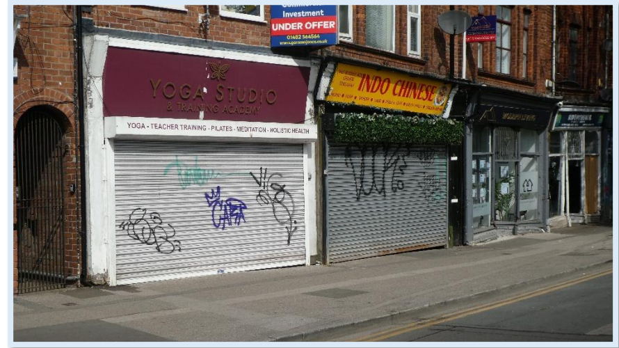
39 - Nos.5-7 - Historic shop front, harmed by the introduction of a roller shutter.
