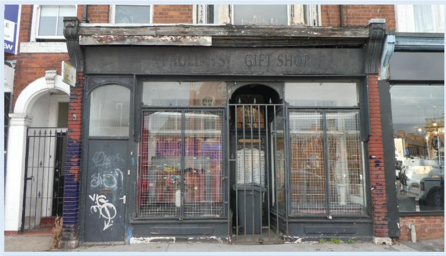
42 - No.77 Princes Avenue, with poor quality grills.
