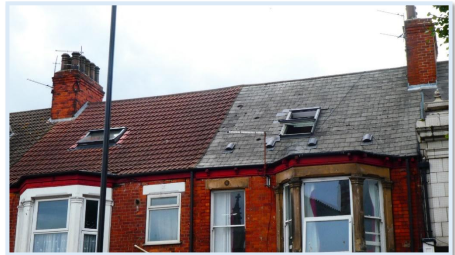
31 - Bay window details, contrasting roof materials and use of roof lights at Nos.79-81.
