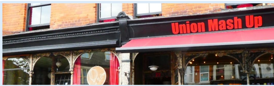
122 - Unauthorised canopies at Nos.22-24.
