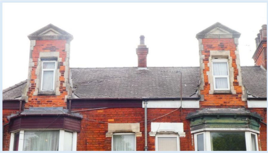
20 - Roof slates and dormers at Nos.51 and 53.
