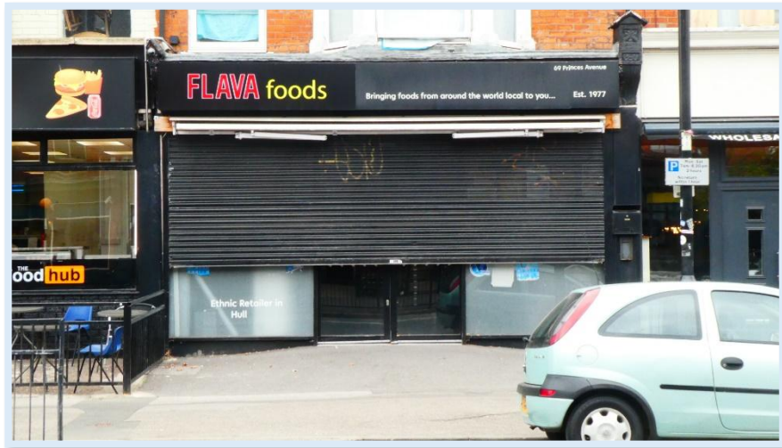
75 - Unauthorised Roller Shutter at No.69.
