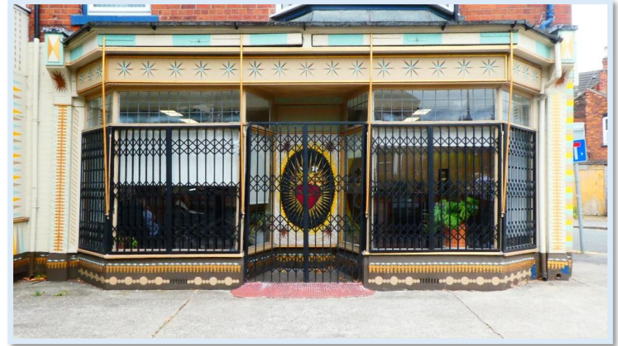
43 - One of the best surviving shop fronts, with retractable awning. Poor quality grills.
