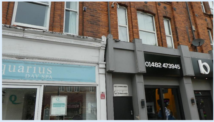
123 - Mis-matched shop front details in Nos.7-43.
